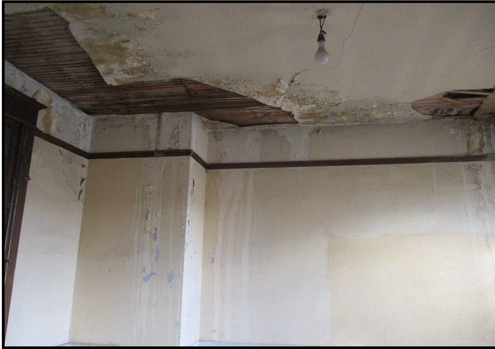
Typical Ceiling with Water Damage
